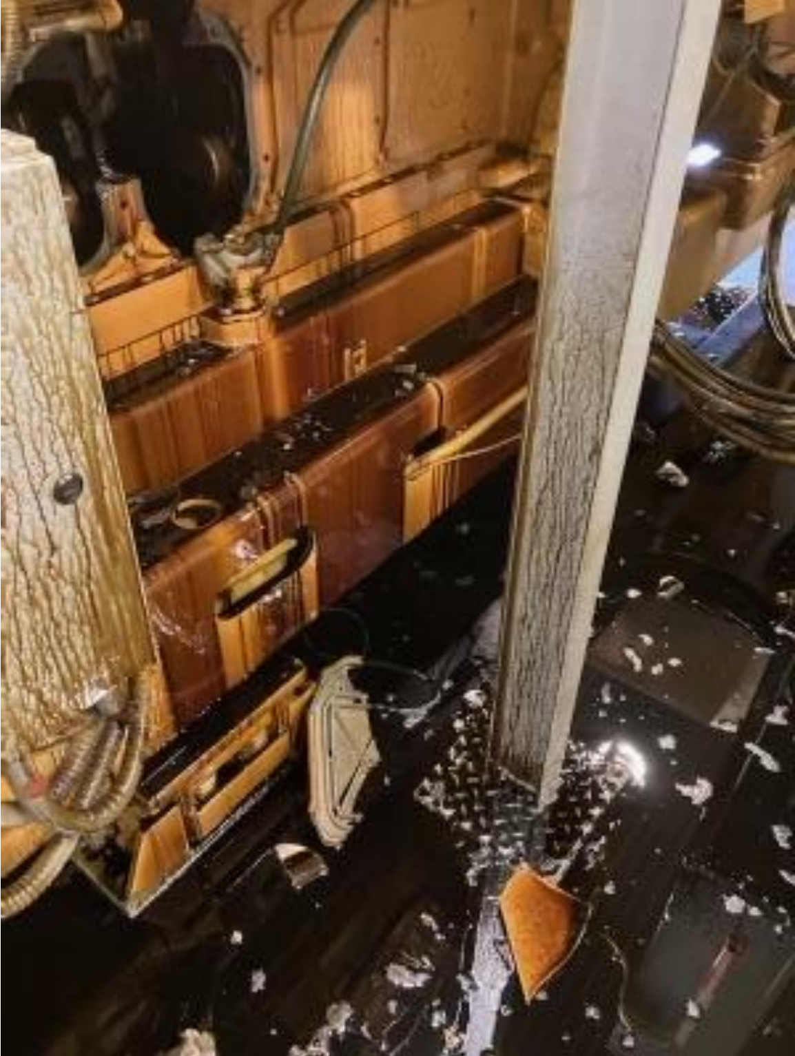
Photo A-5: Large Amount of Lube Oil Spilled onto the Floor due to the Failure; this was Contained Once Power was Restored
