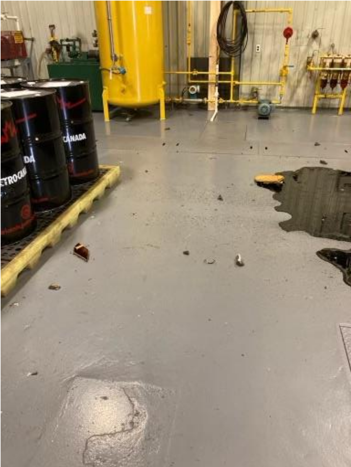
Photo A-4: Pieces of Engine Block Scattered on the Floor with Lube Oil that Spilled from the Engine
